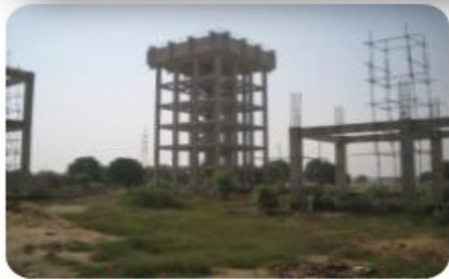
100,000 Gallon Over Head Water Tank
